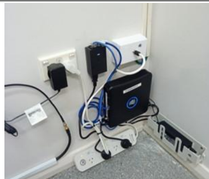
Figure 2: Network Termination Device (NTD) and Power Supply Unit (PSU)
