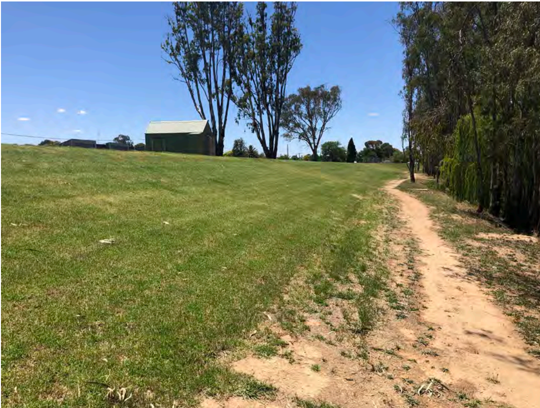
Photo 5: South side of existing levee from observation platform looking east along the proposed pathway. Note the works will formalize the existing track right of frame. Photo: D.Wall
