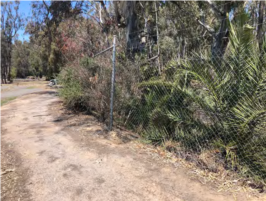
Photo 7: Vegetation management and levee straightening behind the sports oval, east orientation. Works will see the removal of exotic vegetation, existing fence and levee strengthening with fill. Photo: D.Wall
