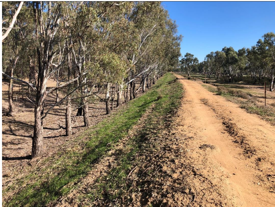
Trees to be removed along the toe of the bank to ensure trees roots do not impact the structural integrity of the levee.
