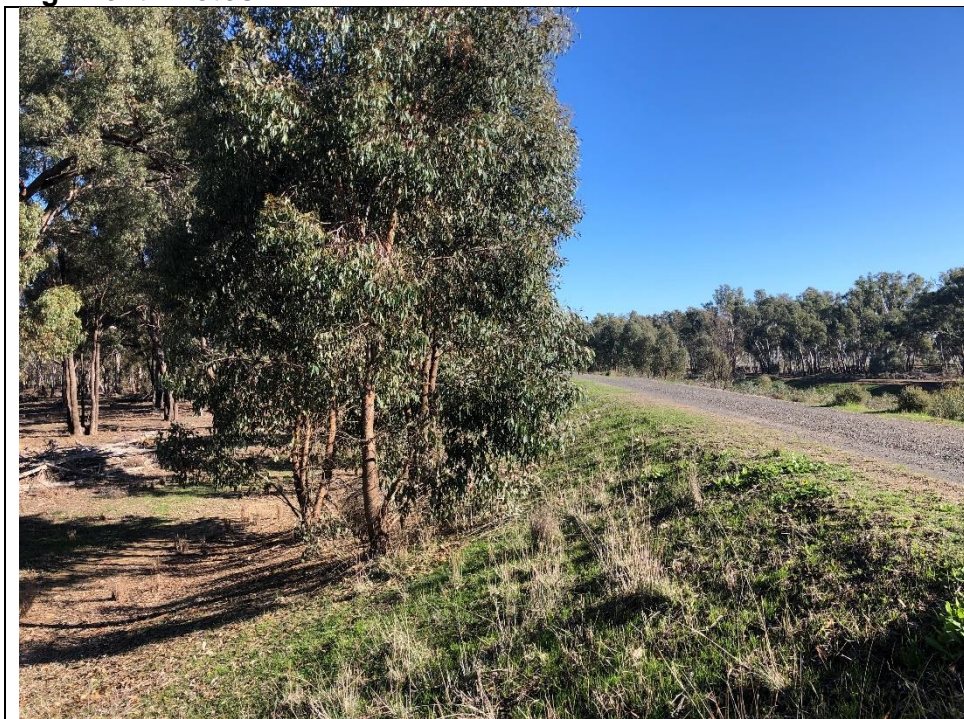
Trees require for removal seen here to remove them from the toe of the bank.
