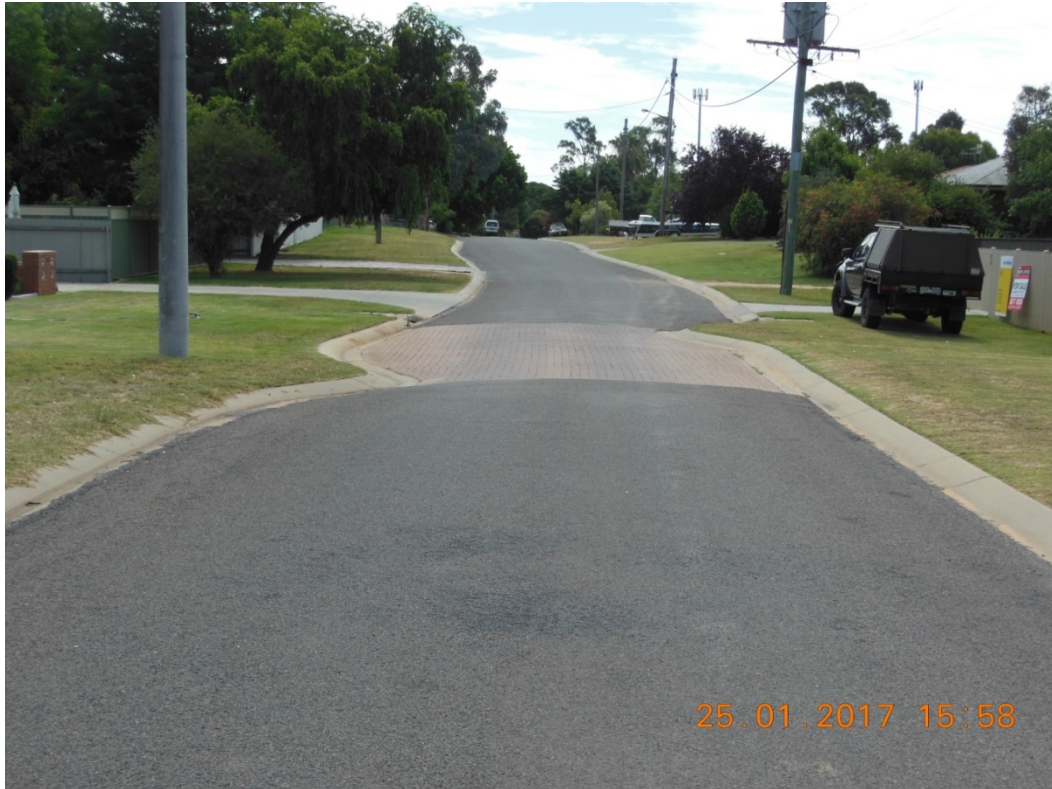
Figure 2 - KAMAROOKA STREET TRAFFIC DEVICE
