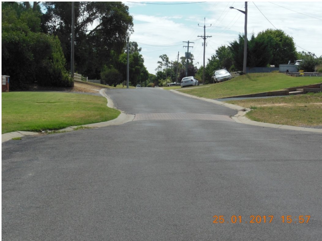
Figure 3 - KAMAROOKA STREET TRAFFIC DEVICE
